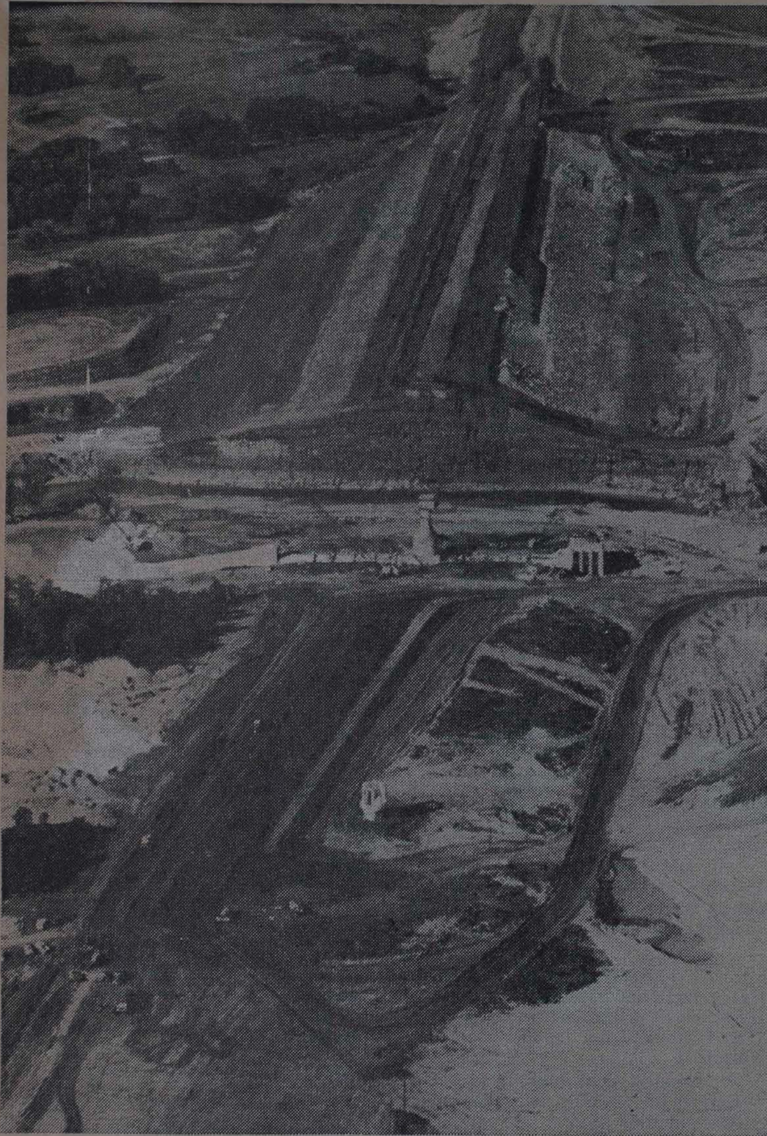
DAM TAKES SHAPE —This view (left) of the Little River dam along its axis from northeast to southwest shows the round spillway inlet (center foreground) and beyond it the outlet works with its gridded inlet (right) and tower for gate control valves. Only the square structure atop the tower will project above the complet-
